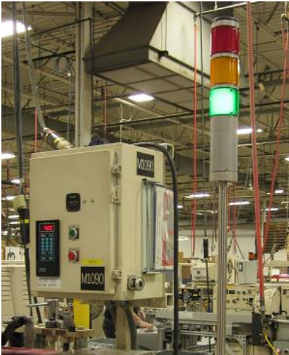
FIG 2: Manufacturing equipment with 3 stack lights
